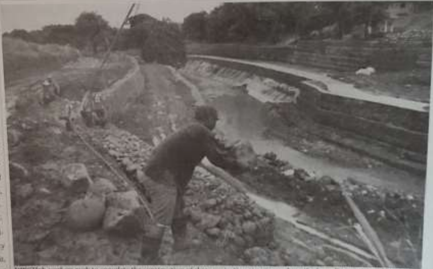
DPW High workers rush to complete the construction of slope protection structures along the Inus River in Daanarinas City, Cavite last July 23. The completion of the project this year is expected to lessen flooding in the cities of Inus and Bacour during rainy season.
